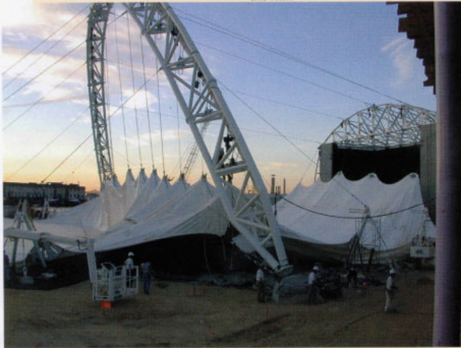
Installation crewmembers prepare to raise and tension the BankBoston Pavilion fabric roof. Design by A.Form Architecture, fabric installation by Span Systems Inc.
